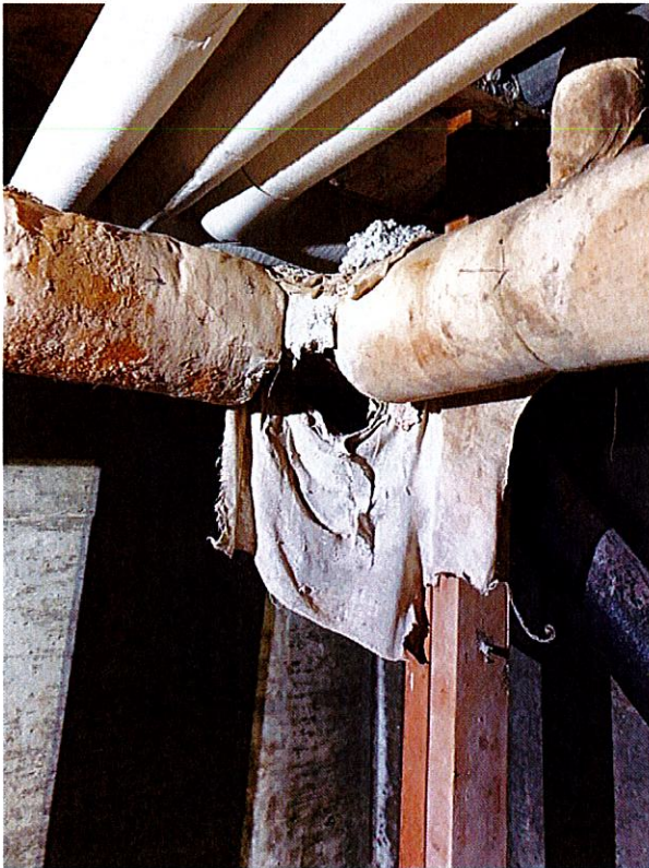
Damaged asbestos fitting
