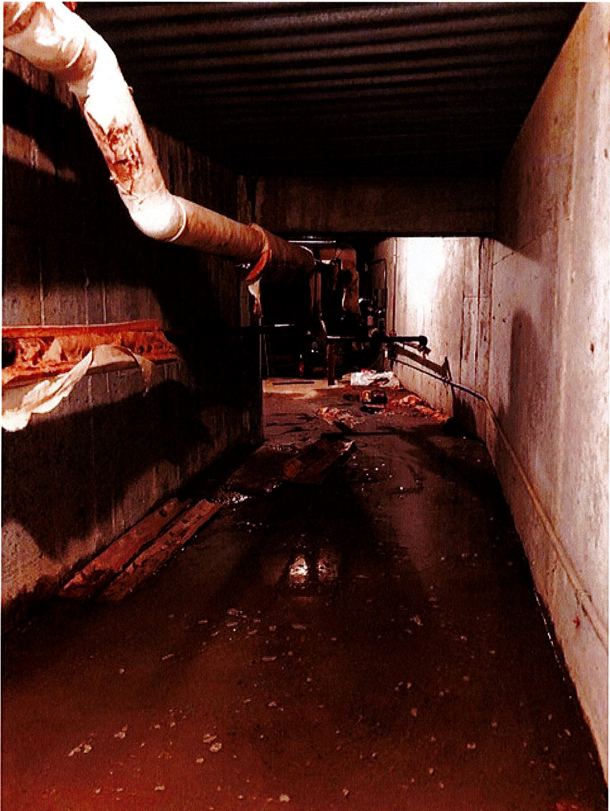
Water on concrete floor
