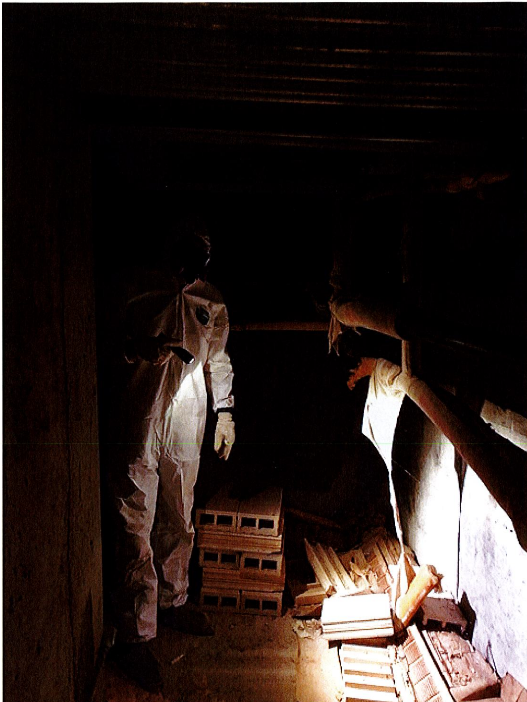
Some contaminated construction materials to be removed
