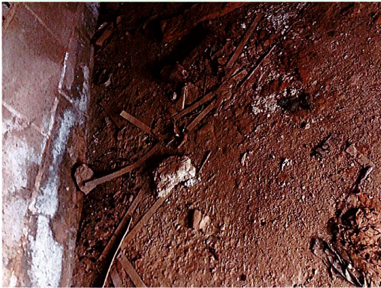
Asbestos Pipe fitting debris
